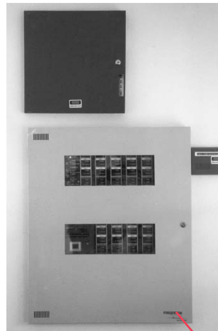
FireSystem 2000 Control Panel
