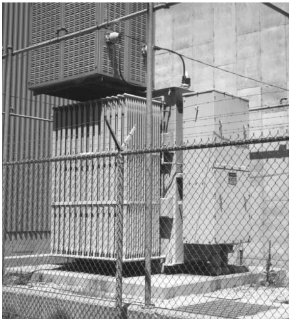
Photos taken at: Monroe Power Plant, Detroit Edison Co., Detroit, Michigan., U.S.A.
